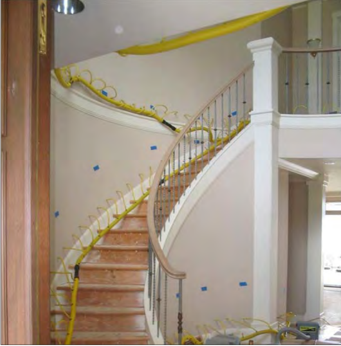
Ceiling and wall dryouts with patented Active Hoseline (tubing can be cut to the length needed for the job)
