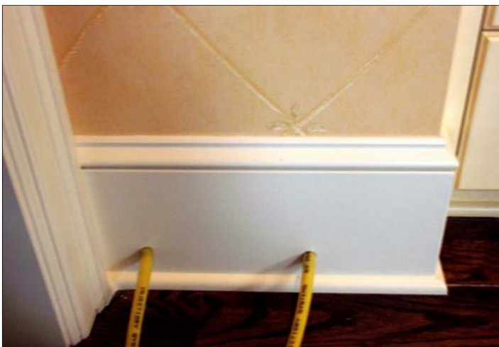
INJ01 drying walls through 1/4" easy to repair holes in baseboard in order to save wallpaper
