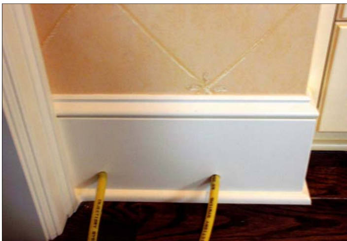
INJ01i drying walls through 1/4" easy to repair holes in baseboard in order to save wallpaper
