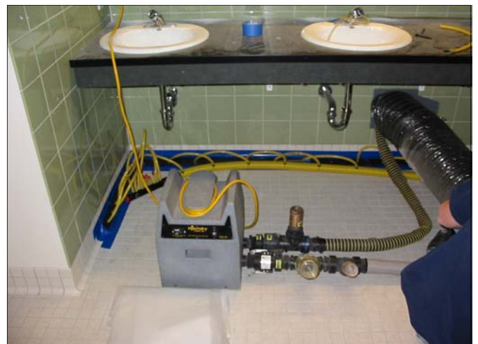
Wall drying behind tile
